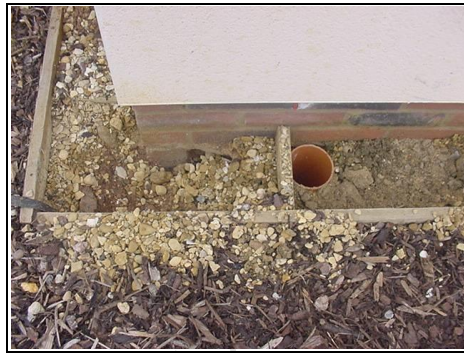
The exposed French Drain which hasn't been traditionally constructed
