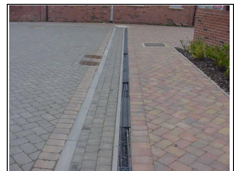
Broken running drain to the rear of the property
