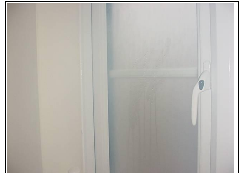
Condensation to window
