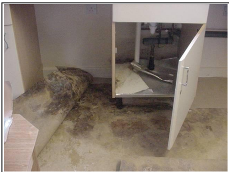
Dampness under kitchen unit
