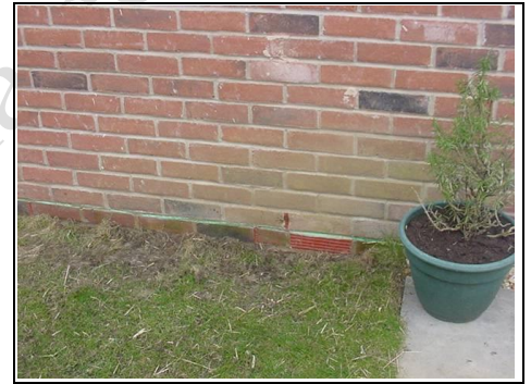
French Drain needed to the rear of the property?
