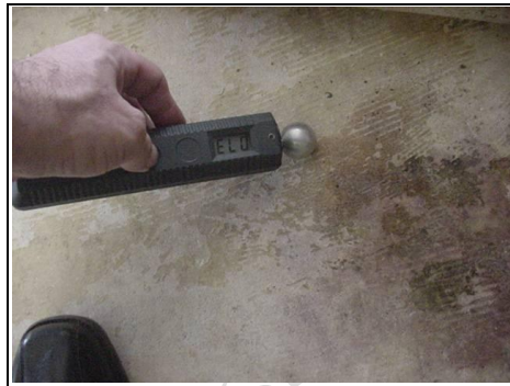
Electronic damp meter readings on kitchen floor
