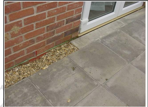
Airbrick acting as a gutter
