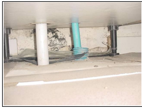
This shows dampness where the floor meets the wall
